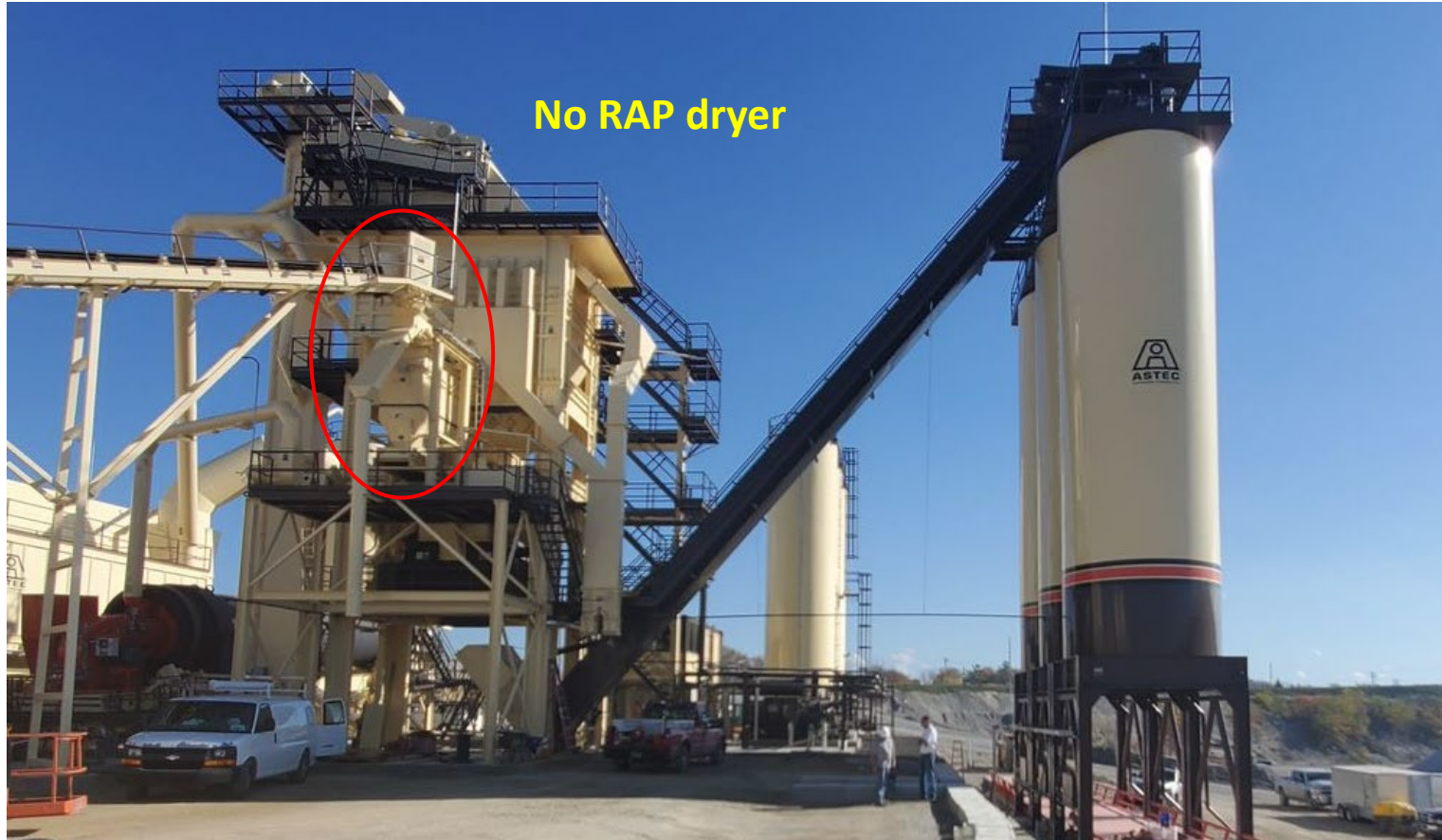
Batch Plant RAP System – USA Style
