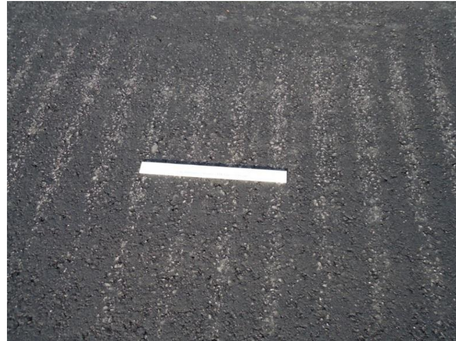
Over or Under- Compaction Can Occur
