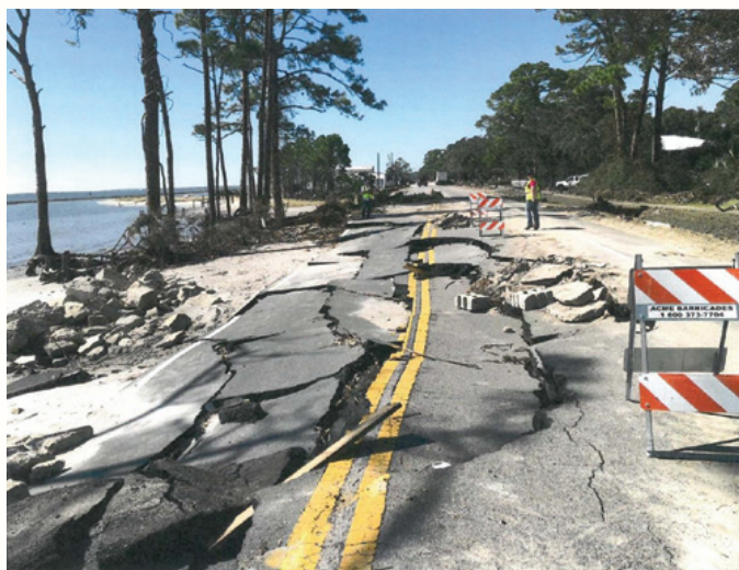
Hurricane Michael damaged SR-30 (US-98) in Franklin County, Florida. Photo Courtesy of Kevin Wall.
