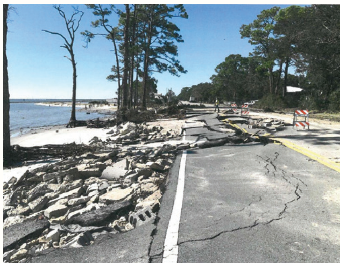
Hurricane Michael damage on SR-30 (US-98) in Franklin County, Florida. Photo Courtesy of Kevin Wall.
