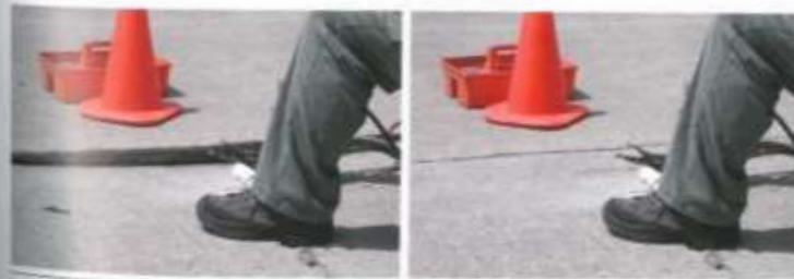
Figure 4.4. Settled slab before (left) and after (right) slab jacking (courtesy of John Roberts, International Grooving and Grinding Association [IGGA])
