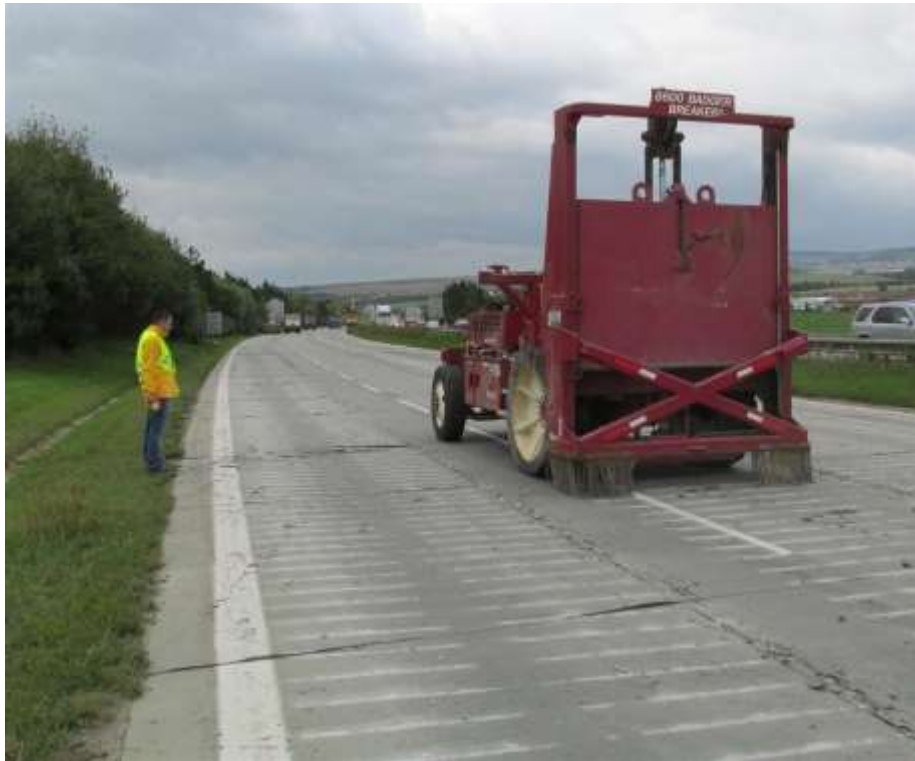
Crack & Seat: used on plain (unreinforced) concrete pavements; crack spacing 1 to 5 ft.
